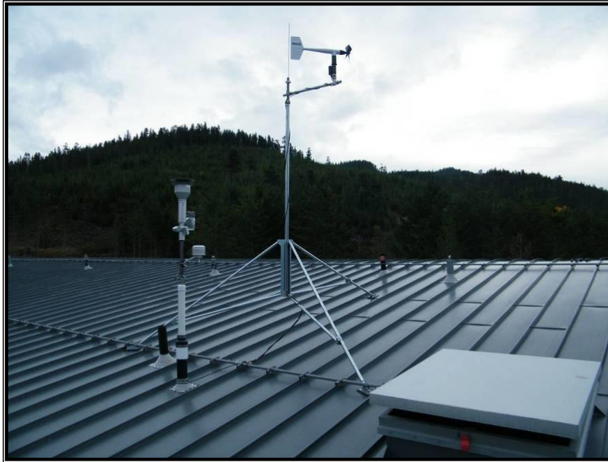
Figure 2-4 Tripod Mounted Anemometer and TEOM Inlet located on the Roof of the HPC building
