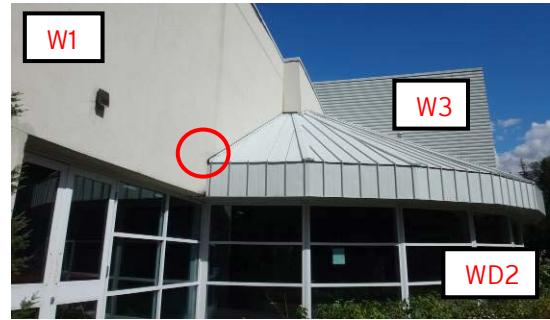
Photo A1-4 Connection between Standing Seam Metal Roof and South Wall of Pool
