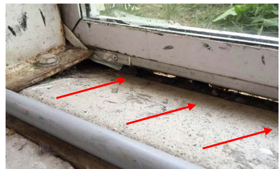
Photo A1-25 Ice Arena - Concrete Curb Deflection
