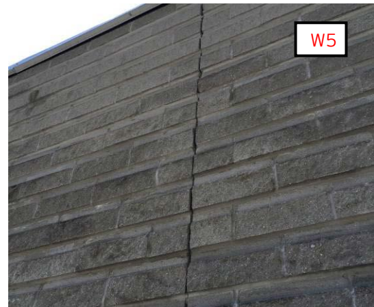
Photo A1-20 Ice Arena - Unsealed Control Joints
