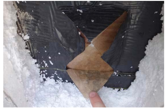
Photo A1-13 Fitness Centre - Northeast Corner - Exploratory Recess No.6
