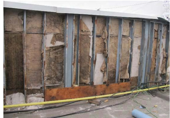
Photo A1-6 Pool Parapet - Deterioration
