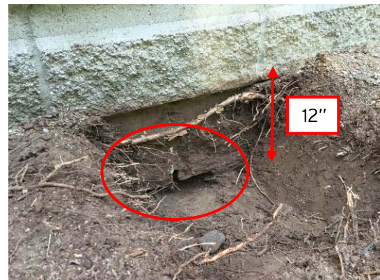
Photo A1-22 Ice Arena - Exploratory Recess No.10
