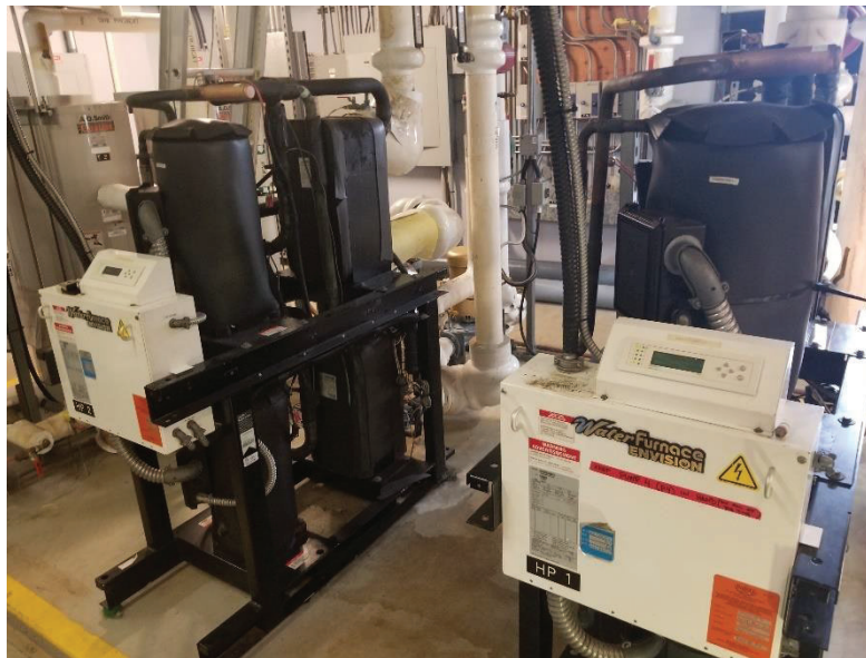
Figure 1: Pool-Side Heat Pump Plant
