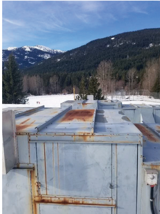
Figure 7: AHU-1 and AHU-2 (Cardio and Weight Room) Site Photo
