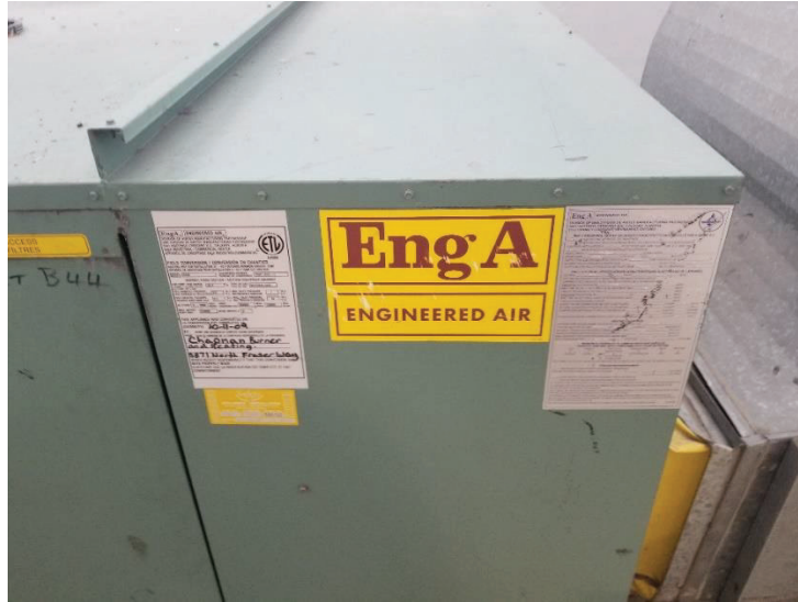
Figure 5: AHU-1 (Lobby Space) Site Photo
