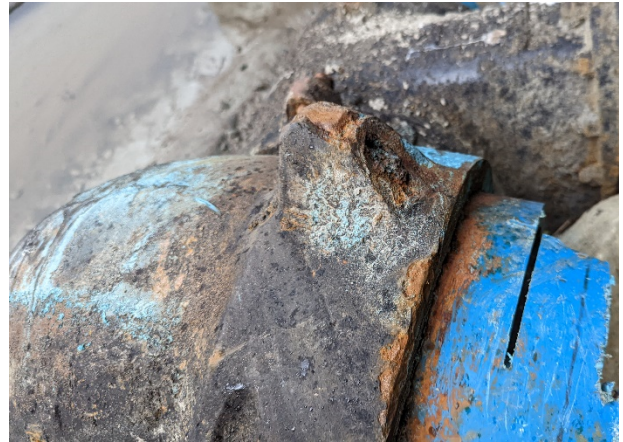
Photo 2 - Corroded 90° Bend Restraining Ear.
