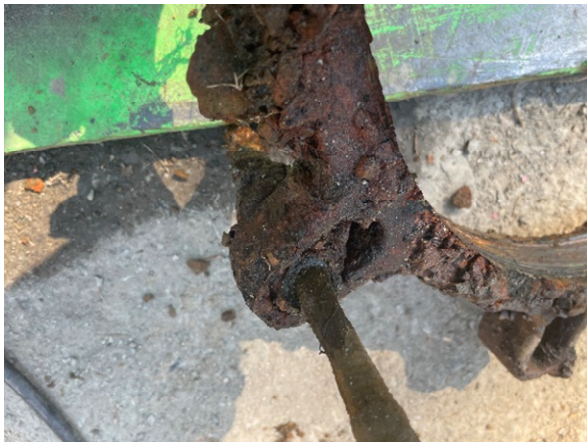
Photo 1 - Corroded Restraining Rod (S1-7 90° Bend)
