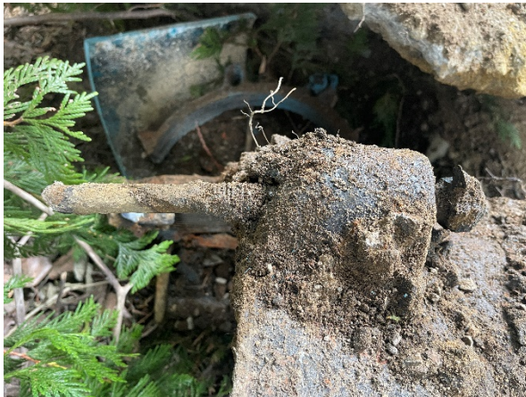
Photo 3 - Corroded Restraining Rod (S1-4 11.25° Bend)
