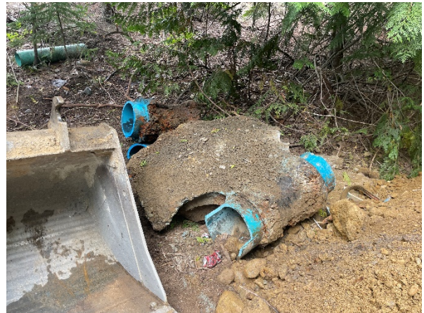
Photo 4 - Encrustation and Surface Corrosion (S1-6 11.25° Bend)
