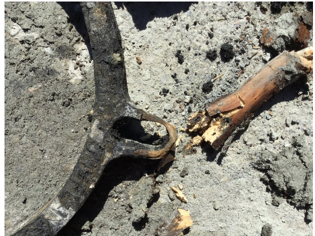
Photo 2 - Corroded Restraining Ring Ear.
