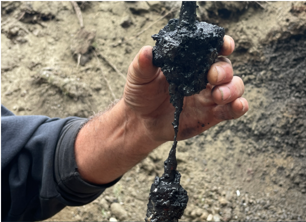
Photo 1 - Corroded Restraining Rod.
