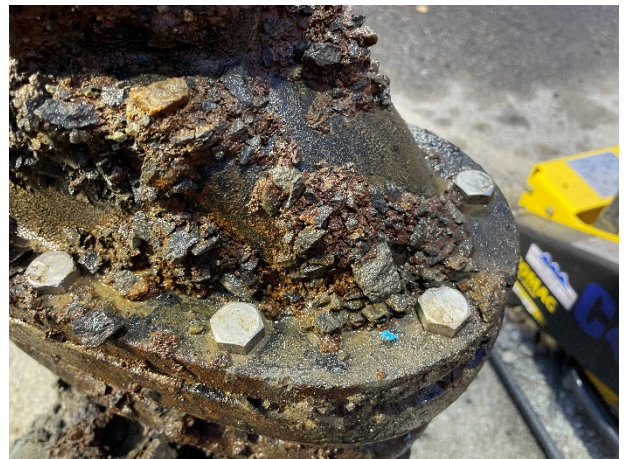
Photo 4 – W1-D Valve Bonnet Bolts
