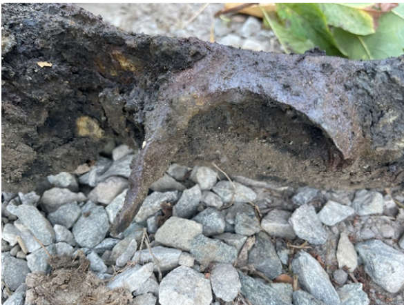
Photo 3 - Corroded Restraining Ring Ear.
