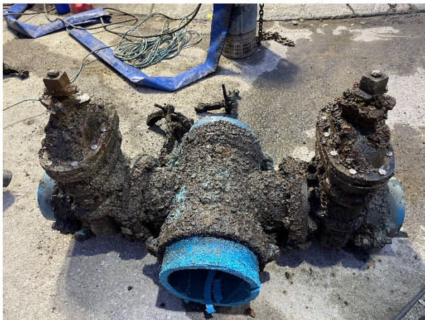
Photo 3 – W1-D Cross and Valves
