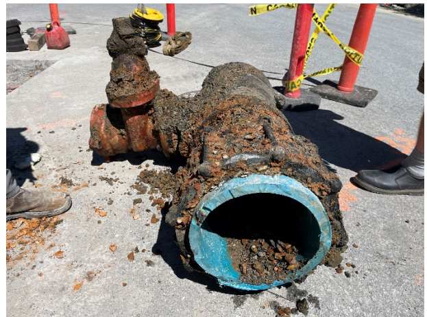
Photo 4 – Valve & Tee Corrosion.
