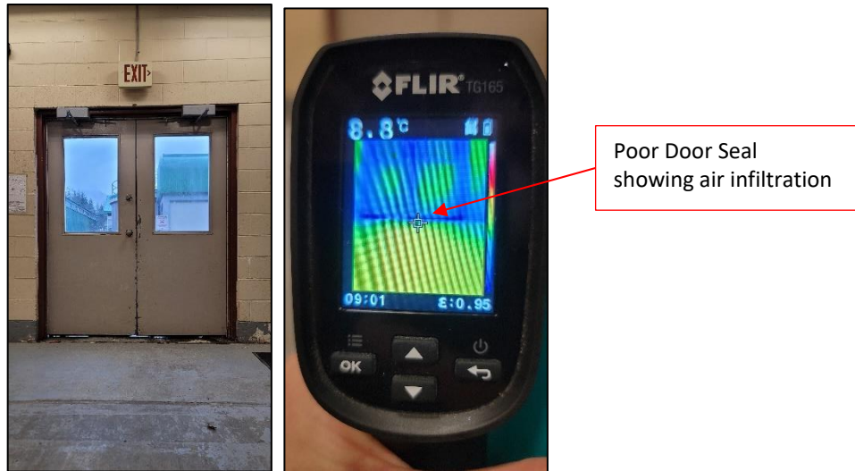
Figure 72: Existing Poor External Door Seals
