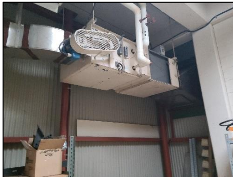
Figure 38: Compressor Room MAU.
