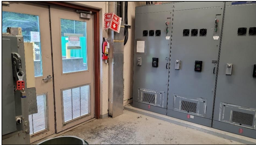
Figure 24: MCC Panels & Door Grilles (close proximity)
