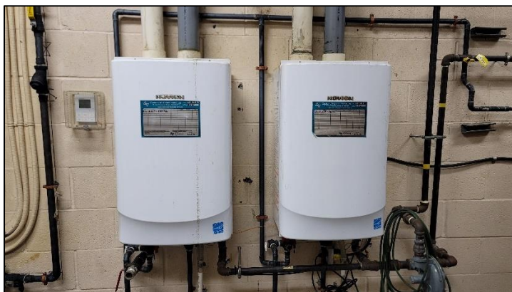
Figure 7: Boilers serving Heating and Service Water
