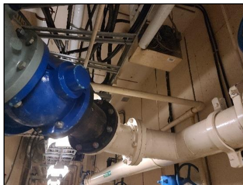
Figure 14: Water Entry Room Unit Heater
