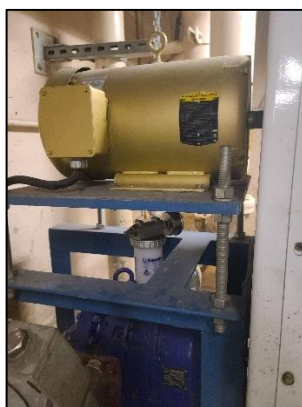
Figure 16: Sludge Pump Motor
