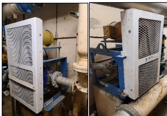
Figure 15: Water Entry Room Sludge Pumps
