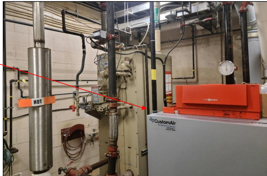
Figure 4: Boilers serving Heating and Service Water
