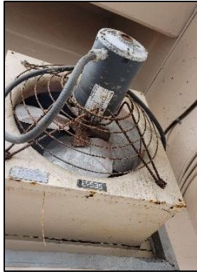
Figure 20: Maintenance workshop exhaust fan
