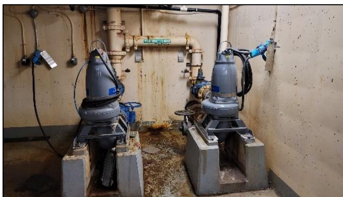
Figure 11: Liquid recycle pumps
