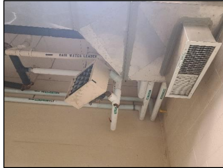
Figure 13: Lower Floor Entrance Unit Heater
