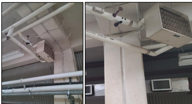
Figure 36: Compressor Room - Unit Heaters (EH254 and EH255)
