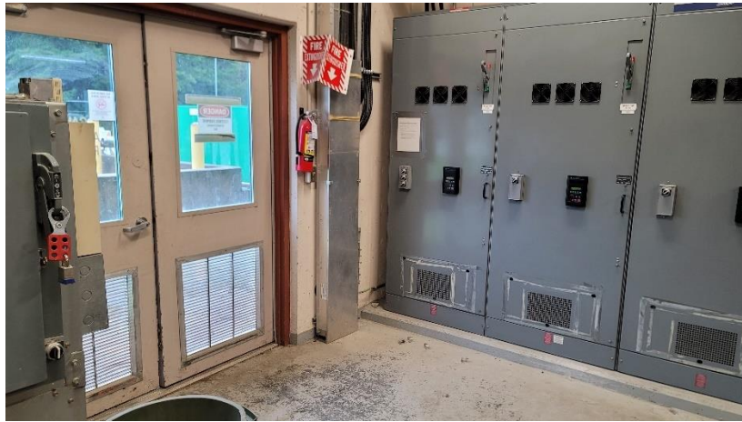
Figure 22: MCC Panels & Door Grilles (close proximity)
