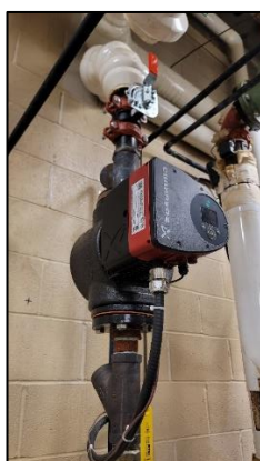
Figure 6: Variable Speed Heating Pumps (PR242)
