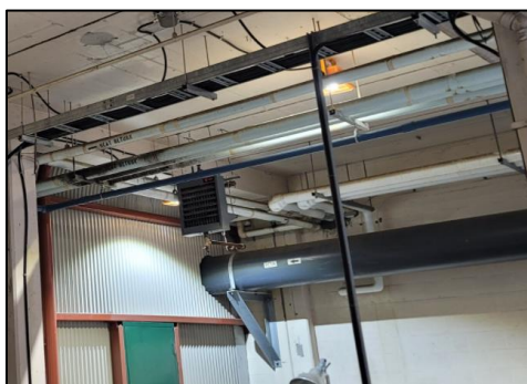
Figure 31: Headworks Area unit heater
