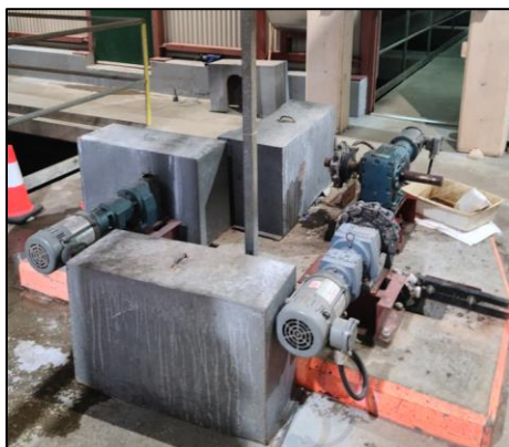
Figure 30: Headworks' area motors.
