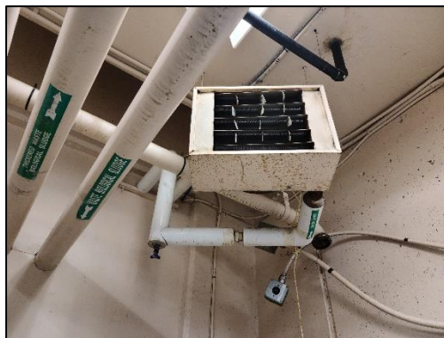
Figure 90: Existing Unit Heater
