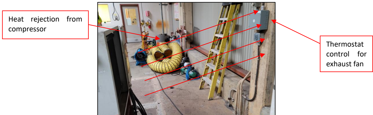
Figure 40: Compressor and Thermostat
