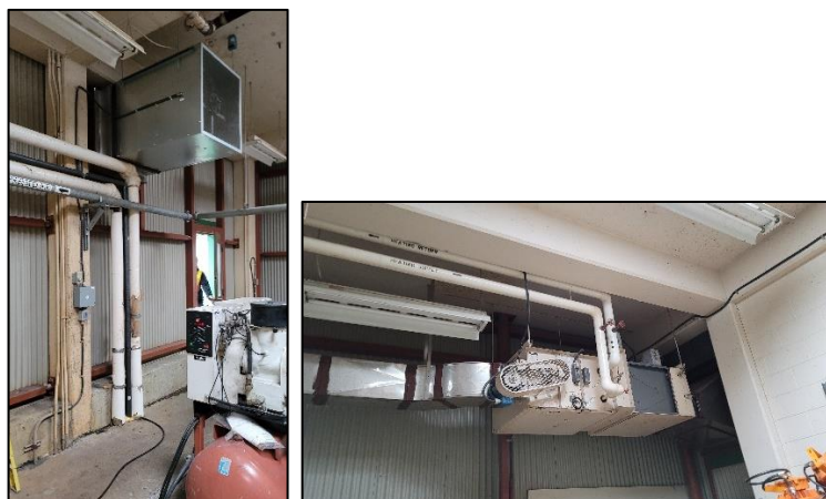
Figure 103: Compressor Room Exhaust Fan and SF245
