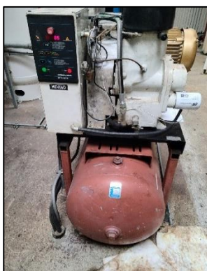
Figure 35: Compressor and motor
