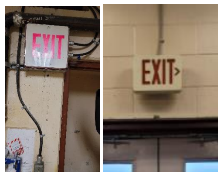
Figure 50: LED Emergency Exit Sign
