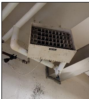
Figure 22: Storage/Safety room unit heater
