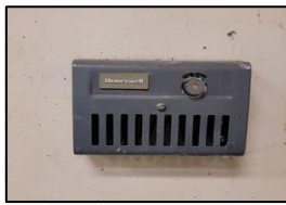
Figure 44: High Setpoint Thermostat
