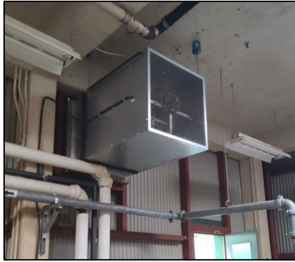
Figure 39: Compressor Room Exhaust Fan.
