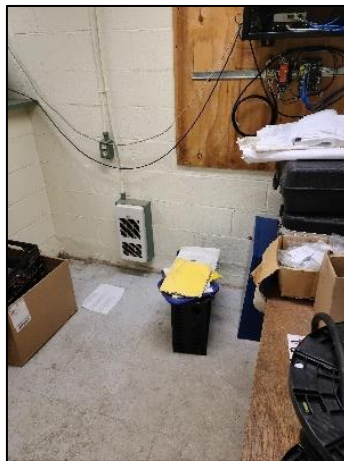
Figure 21: Electrical workshop unit heater
