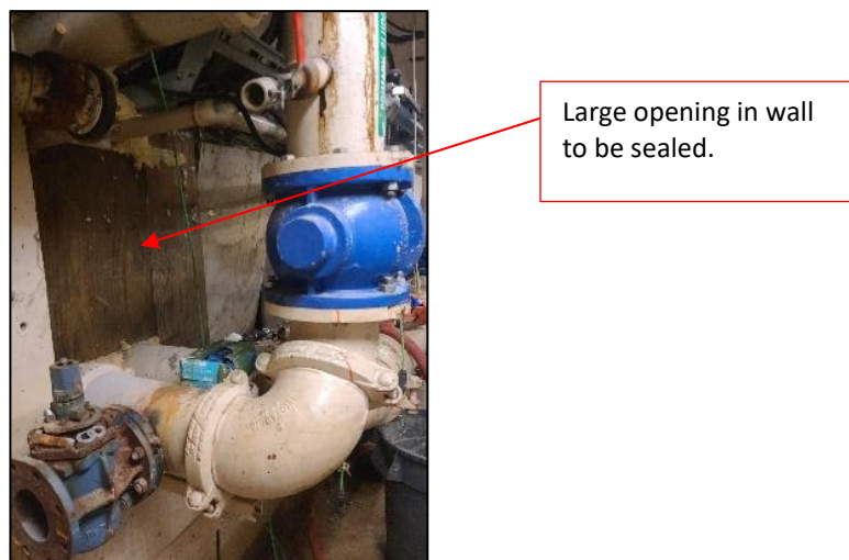
Figure 73: Water Entry Room - Wall Penetration
