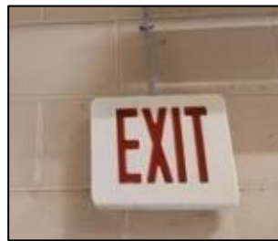
Figure 52: Broken LED Exit sign.
