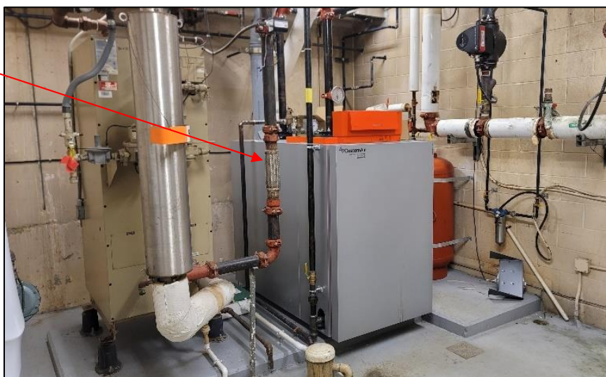
Figure 3: Boilers serving Heating and Service Water
