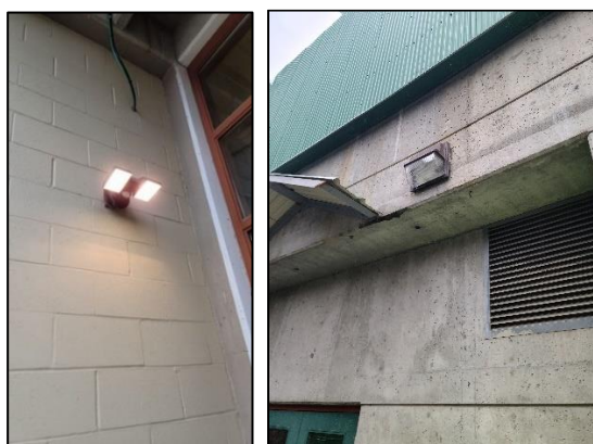
Figure 49: Typical Exterior Lightings.
