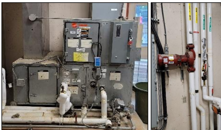
Figure 23: AHU – 4172 & Raw Water-Cooling Loop (Decommissioned)
