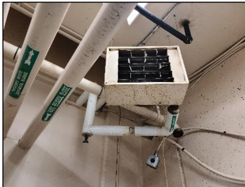
Figure 19: Maintenance workshop unit heater
