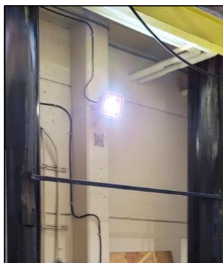
Figure 84: Existing LED-40W-Flood Light
