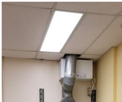
Figure 82: Existing T8-32W-2L-4' Luminaires
