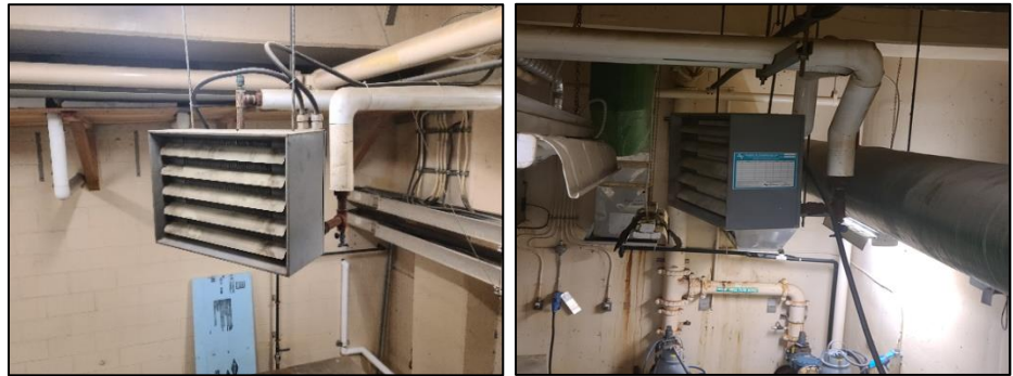
Figure 8: Hydronic Unit Heaters
