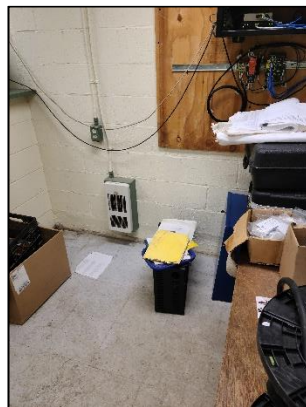
Figure 78: Existing Electric Baseboard
