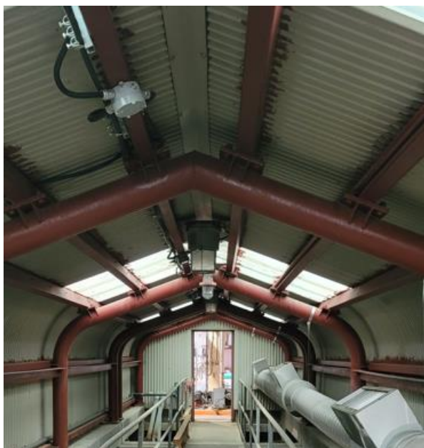
Figure 87: Existing Tunnel lighting
