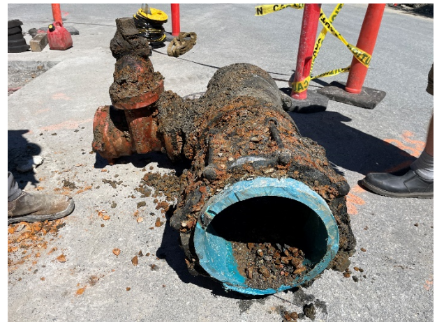
Photo 4 – Valve & Tee Corrosion.
