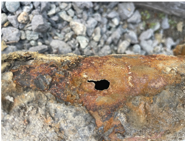
Photo 3 – Blow-off Pipe Corrosion.
