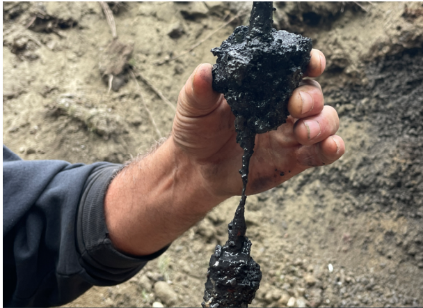
Photo 1 - Corroded Restraining Rod.
