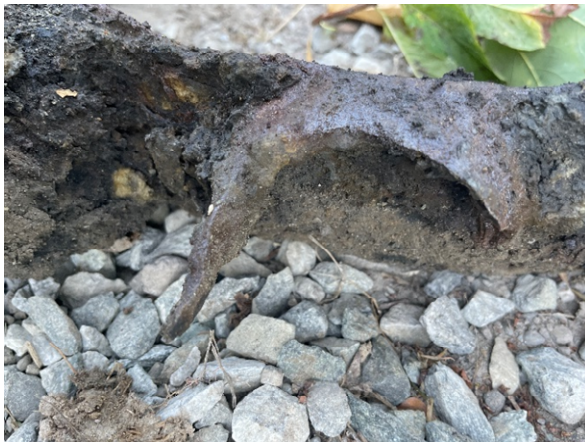
Photo 3 - Corroded Restraining Ring Ear.
