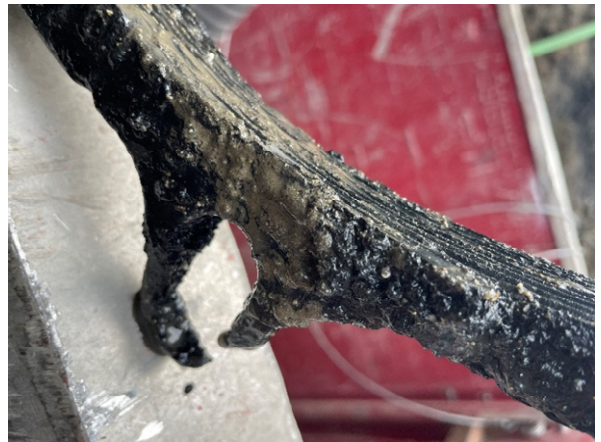
Photo 4 - Corroded Restraining Ring Ear.
