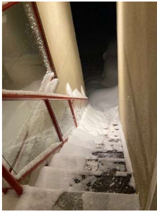
Figure 1 Photo of snow accumulation on exterior stairs leading to front door.
