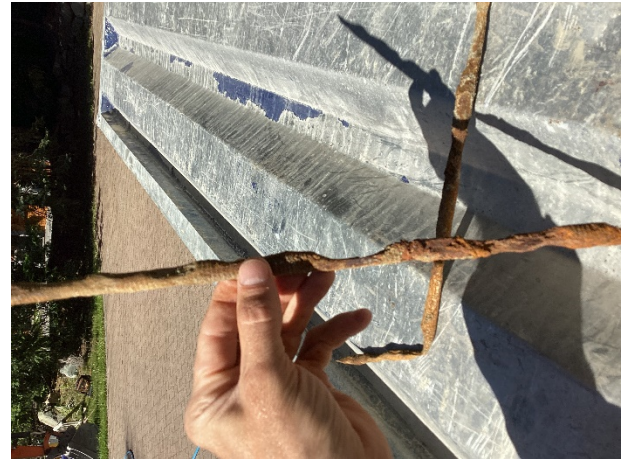
Photo 2 - Corroded Restraining Rod (W4-23 Hydrant Lead)
