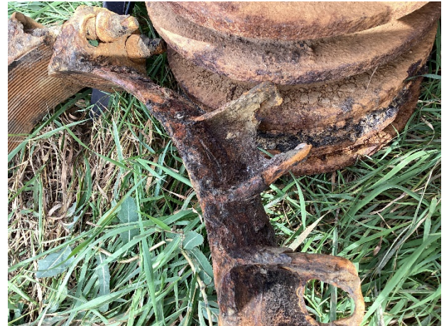
Photo 4 - Corroded Split Ring Restraining Ear (S2-19 22.5° Bend)
