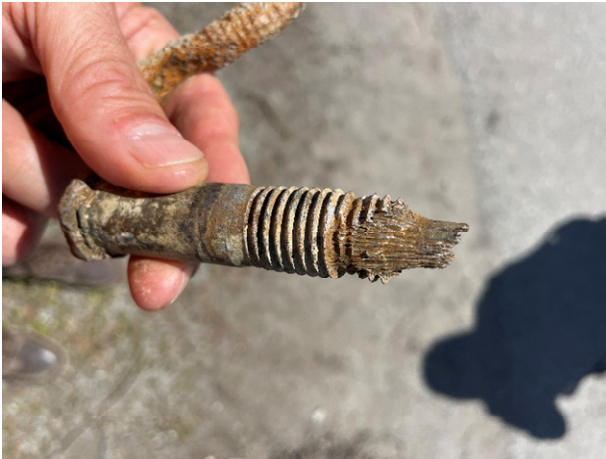
Photo 1 - Corroded Flange Connection Bolt (W4-23 Hydrant Tee)
