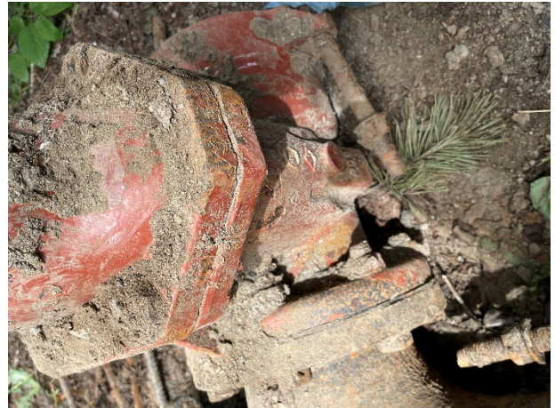
Photo 2 – Minor Surface Corrosion Hydrant Valve W1-18
