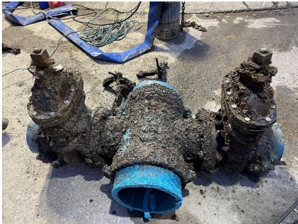
Photo 3 – W1-D Cross and Valves
