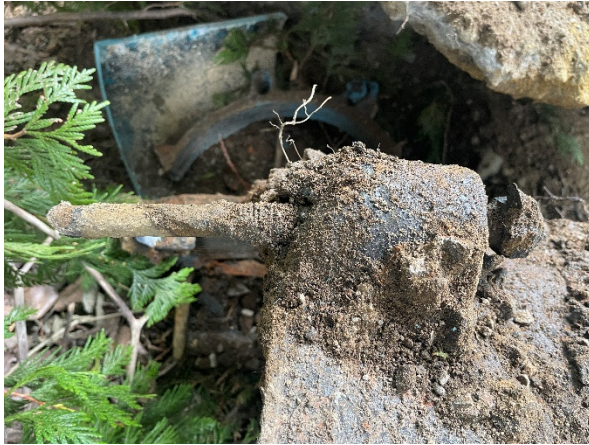
Photo 3 - Corroded Restraining Rod (S1-4 11.25° Bend)
