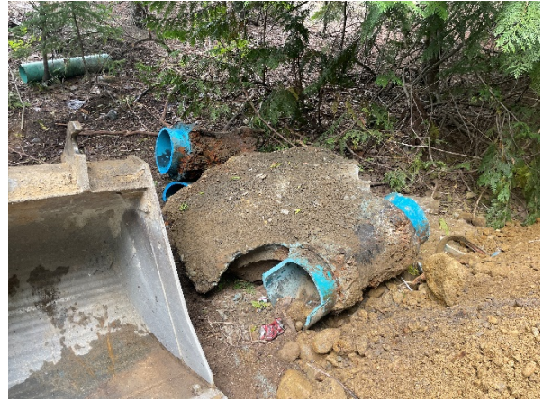
Photo 4 - Encrustation and Surface Corrosion (S1-6 11.25° Bend)
