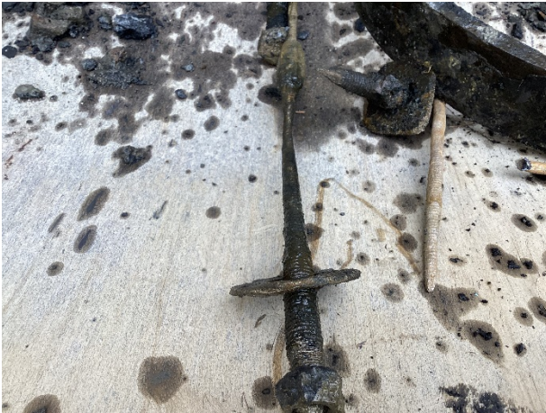
Photo 3 - Corroded Restraining Rod (S2-14 22.5° Bend)
