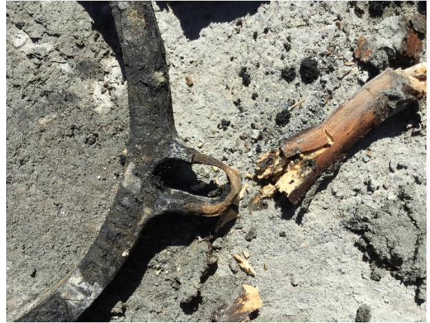
Photo 2 - Corroded Restraining Ring Ear.
