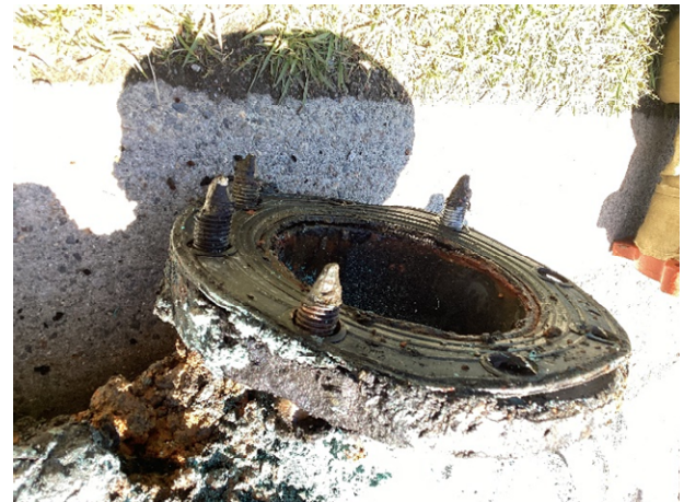
Photo 4 - Corroded Flange Connection Bolts (W4-25 Hydrant Tee)
