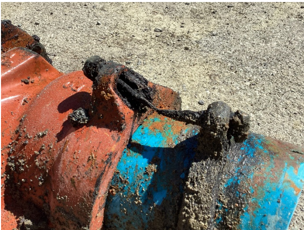
Photo 3 - Corroded Restraining Rod (W4-25 Hydrant Tee)
