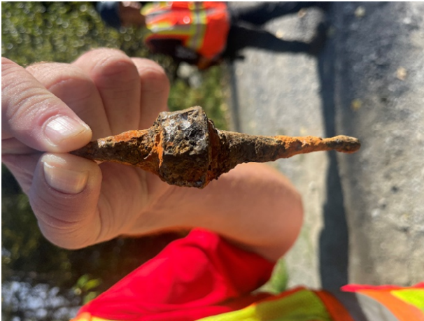
Photo 1 - Corroded Restraining Rod (S2-13 45° Bend)
