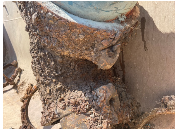
Photo 2 – Encrustation and Surface Corrosion (S1-7 90° Bend)
