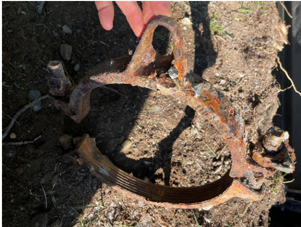
Photo 1 – Minor Surface Corrosion on Restraining Ring W1-17
