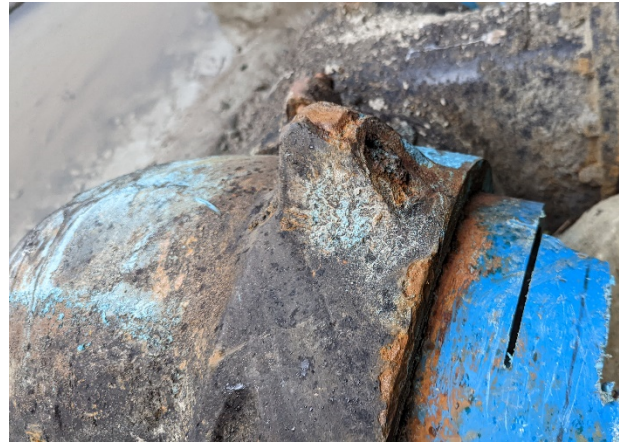
Photo 2 - Corroded 90° Bend Restraining Ear.
