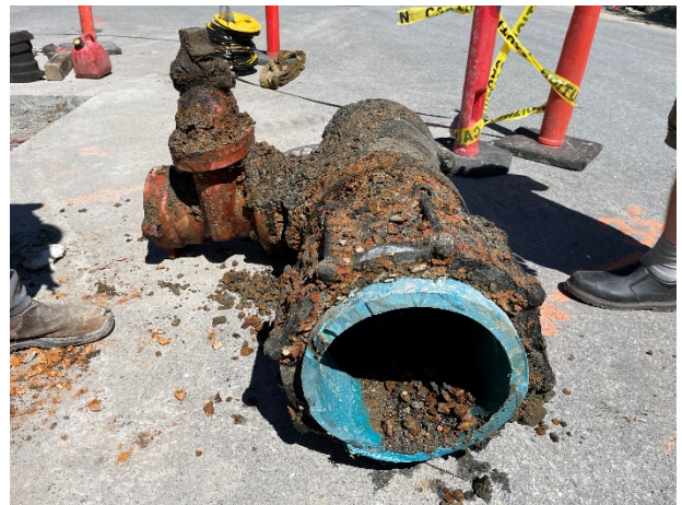
Photo 4 – Valve & Tee Corrosion.
